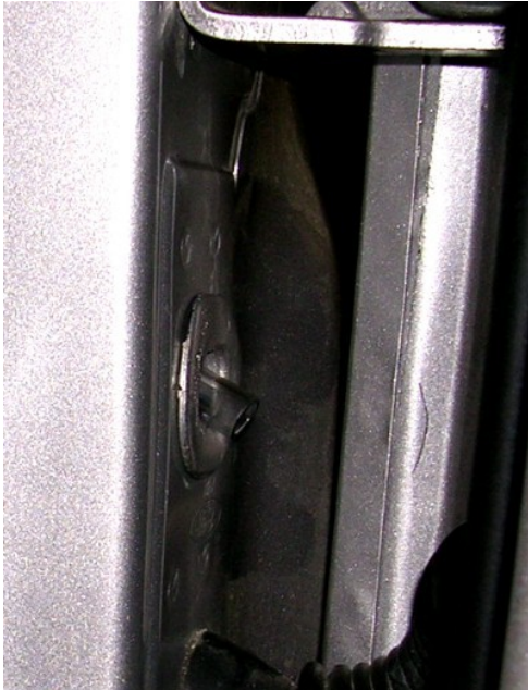
The water drain tube exits through a hole that already existed in the B-pillar framework.
